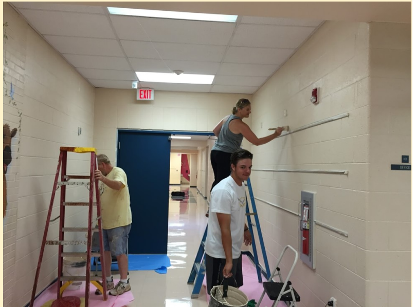
Pictured above are First Baptist of Andersonville members Richard Stretch, Tanya Elkins, and Chase Elkins painting the inside hallways of Andersonville Elementary School.
